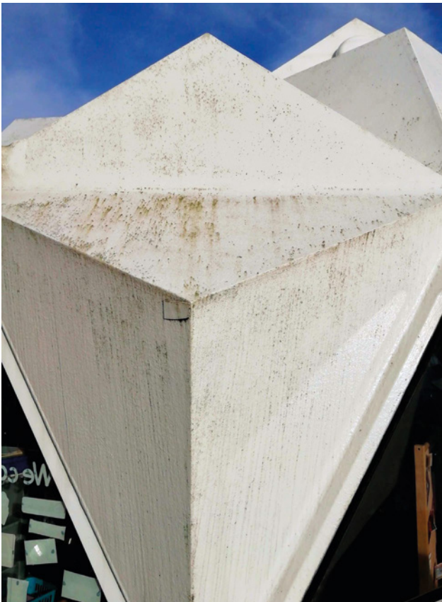
08 The classroom panels in February 2019 before cleaning. A build-up of dirt and algae is trapped in the fibres of the new reinforced polymeric coating. © S. Pritchard
