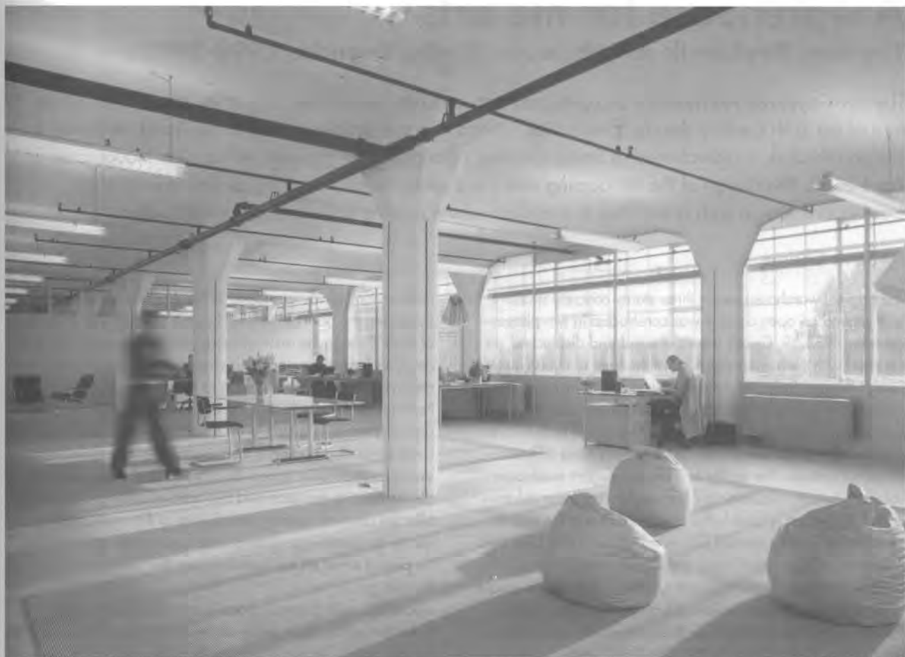
Summer 2001, tenants move in to explore their new work space on 'Coffee Three'. The 1960s sprinkler-system retained the colour according to the original colour-code for systems throughout the factory complex. Photo: Sybolt Voeten architectuurfotografie.
