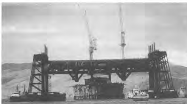
Ninian Central platform November 1977. The 160 m high concrete base is sunk in deep water with 1.3 m freeboard exposed, the steel deck floated over it and the base carefully lifted to mate with the deck. Photo courtesy of Chevron UK.
