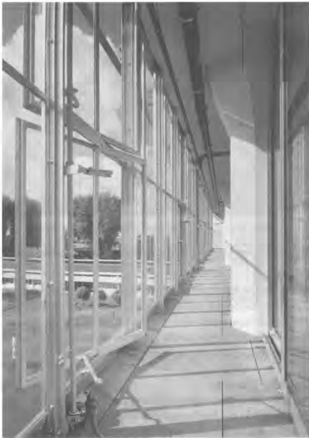
Inside the climate-regulating wall. At the left bottom one of the motors that act upon the vertical rods to operate the vents. Photo: Sybolt Voeten architectuurfotografie.
