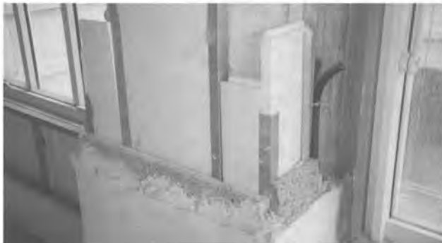
The adopted thermal insulation strategy implied all concrete parts in the facade to be covered by insulation foam and plastered heraklith, losing the original texture and detailing of the structure. Photo: W. de Jonge.
