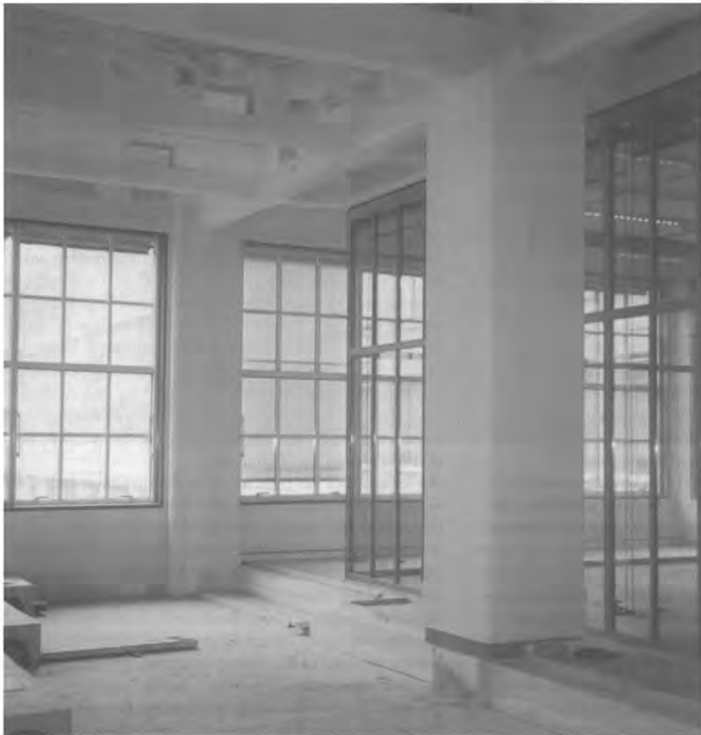
Mock-up of third phase interiors, showing false ceilings, double floors, and glazed partitions. Left, one of the tested 'computer floor' systems. Photo: W. de Jonge.
