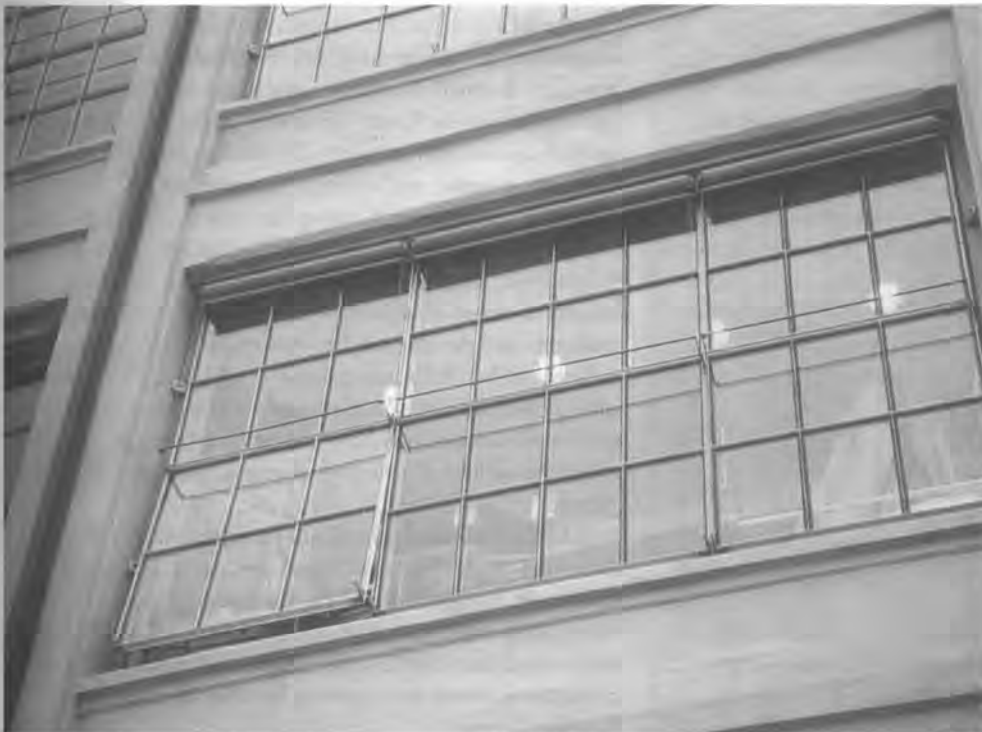
Renzo Piano's beautiful design of the replacement windows, intelligently integrating vision panels, vents and sunscreens, but featuring 4x10 panels in a different proportion. Photo: W. de Jonge.
