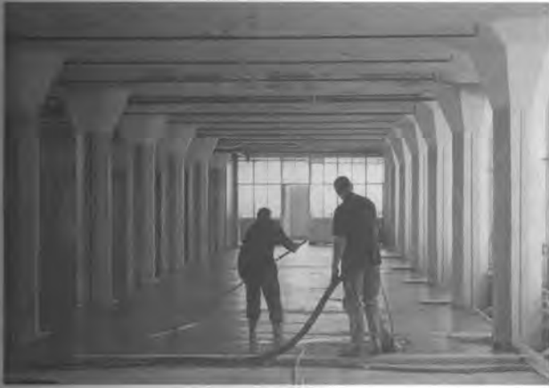
After the instalment of the flat ventilation and cable ducts, a new floor topping is applied. Photo: Fas Keuzekamp.
