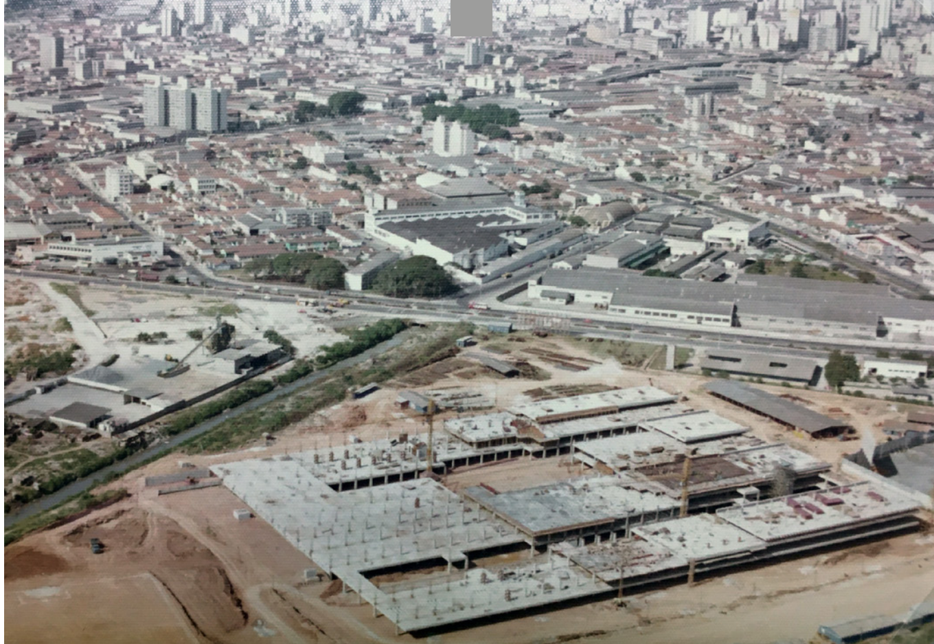
01 Santa Casa Teaching Hospital: The gigantic structure under construction, early 1970s. © Fábio Penteadó's Archive, 2022.
