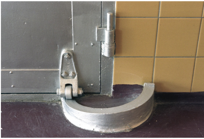
06 Example of the photographic documentation in the archive, showing the 'automatic' self-closing mechanism of a fire door. © Fas Keuzenkamp, 2007, coll. WDJArchitecten.
