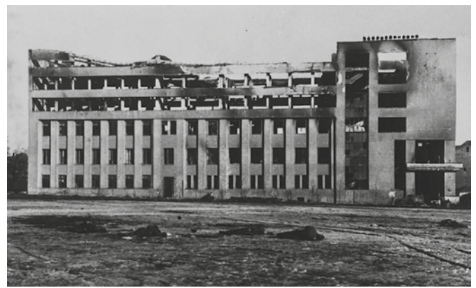
05 The building of the Central Committee during WW2. © Photo from the authors archive, 1944.
