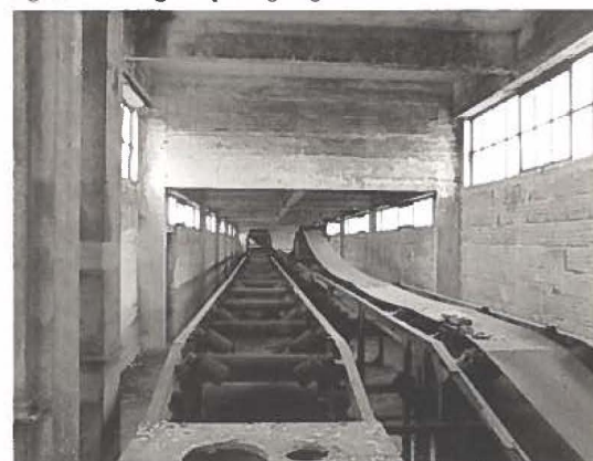
Fig. 3: Moving carpets giving access to the cells
