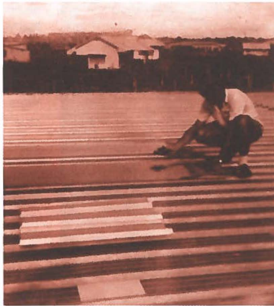
figs. 2-3. Comparisons of reflectance values for weathered and un-weathered asbestos cement and aluminum roof sheets using a photographic exposure meter. Recorded April 1960, architects. Godwin and Hopwood
