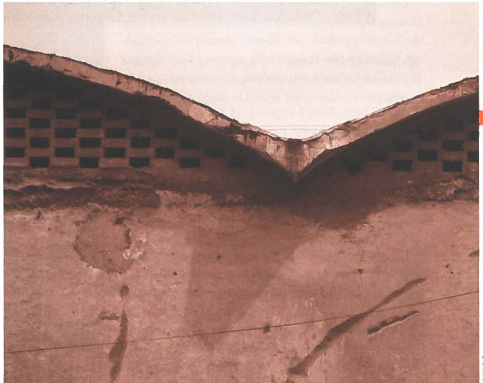
Fig. 1. Auguste Perret , Hamelle warehouses , Rabat's road, Casablanca, c.1920, detail of thin reinforced concrete vaults (first experimented in the Wallut warehouses).
