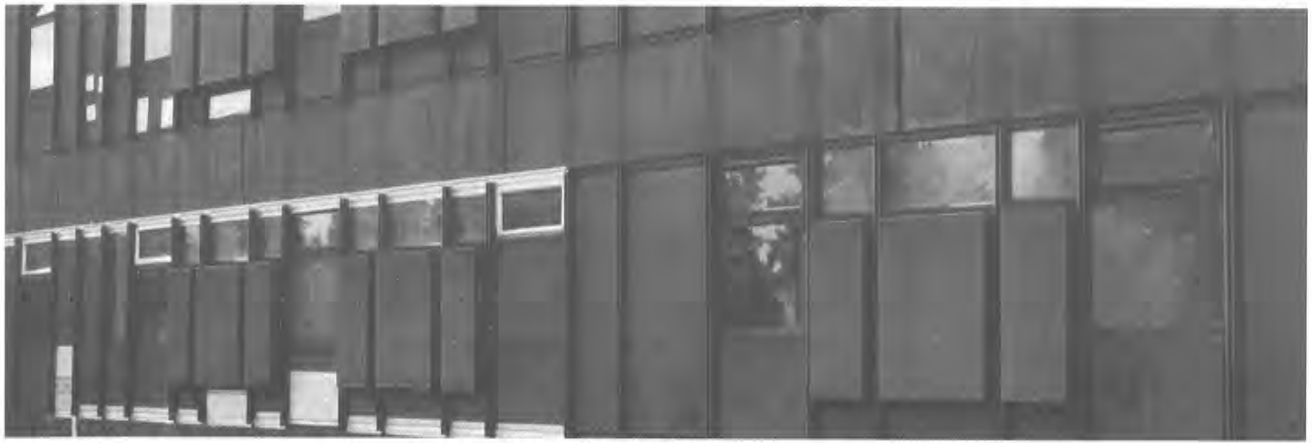
The original Corten steel facade. Period photo: by courtesy of DOCOMOMO Italia Giornale.
