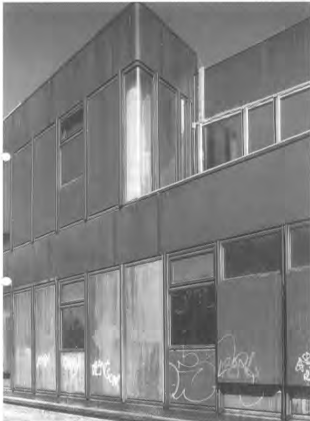
Facade detail prior to restoration, showing Corten steel distress and corrosion-etch streaking on the glazing panels.
