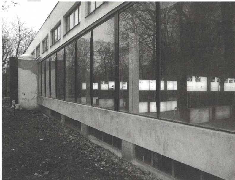
The two illustrations show the north elevation of the Library with the original propositions regained but the rendering still delapidated
