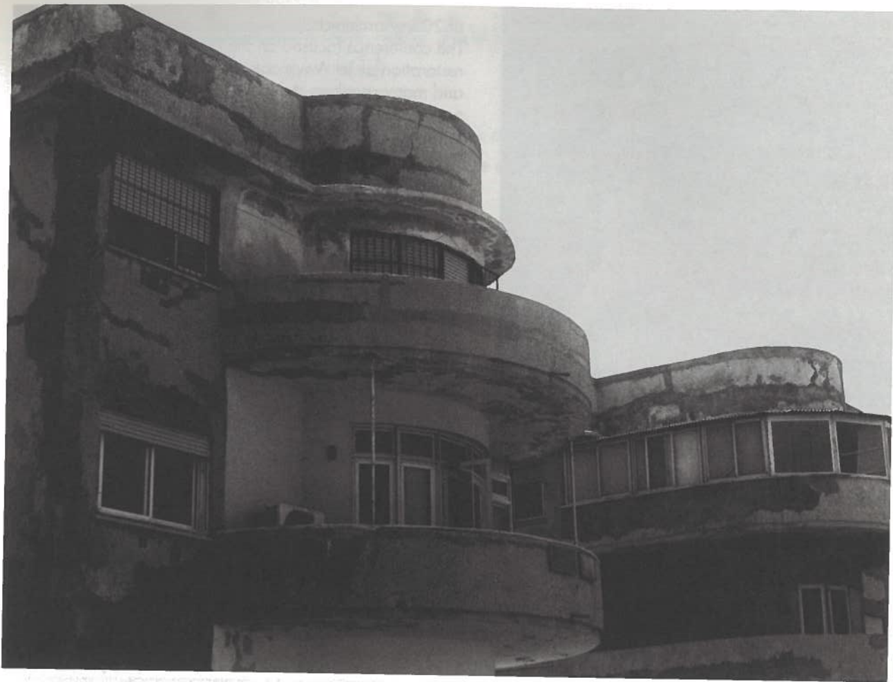
The Reisfeldt House by Pinhas Bizonsky (1935) waits for full restoration after principal concrete repair.
