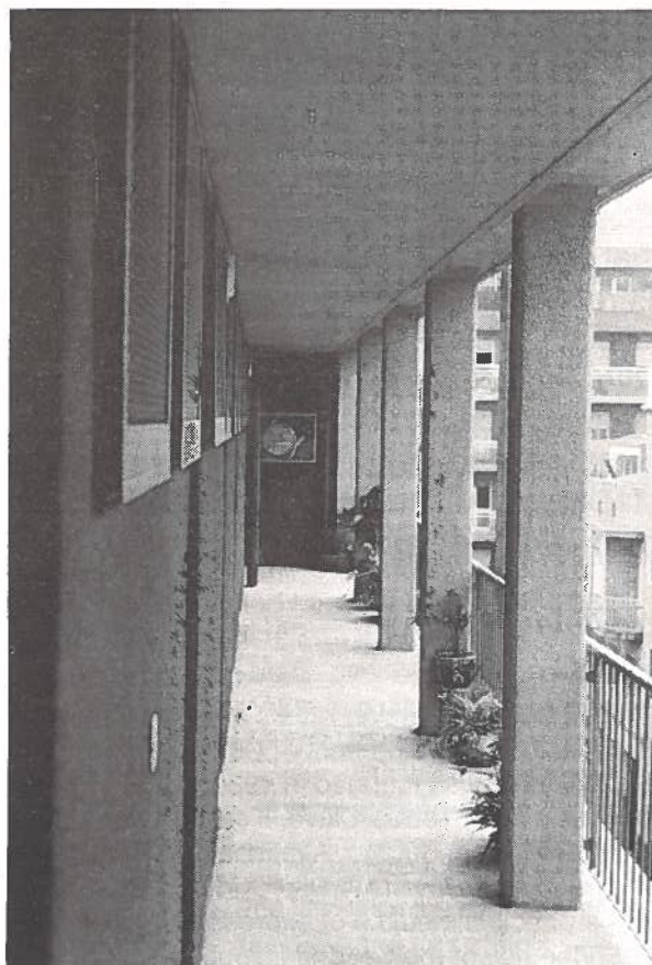
Top and far right: one of the galleries, after restoration. The false ceiling, hiding the new service systems, has been kept quite distant from the facade so as to retain the appearance of the bottom detail of the facade surfaces, as is seen in the right picture. Photos: unknown. Right, top to bottom: section, 1st floor plan, 2nd floor plan and section (upside down) of the restoration project.
