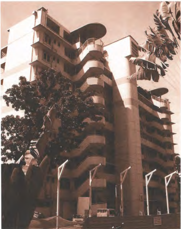
Fig. 4. High-rise SIT apartment building in Upper Pickering Street (next to Hong Lim Park) in the process of demolition (this picture was taken on May 25, 2003)
