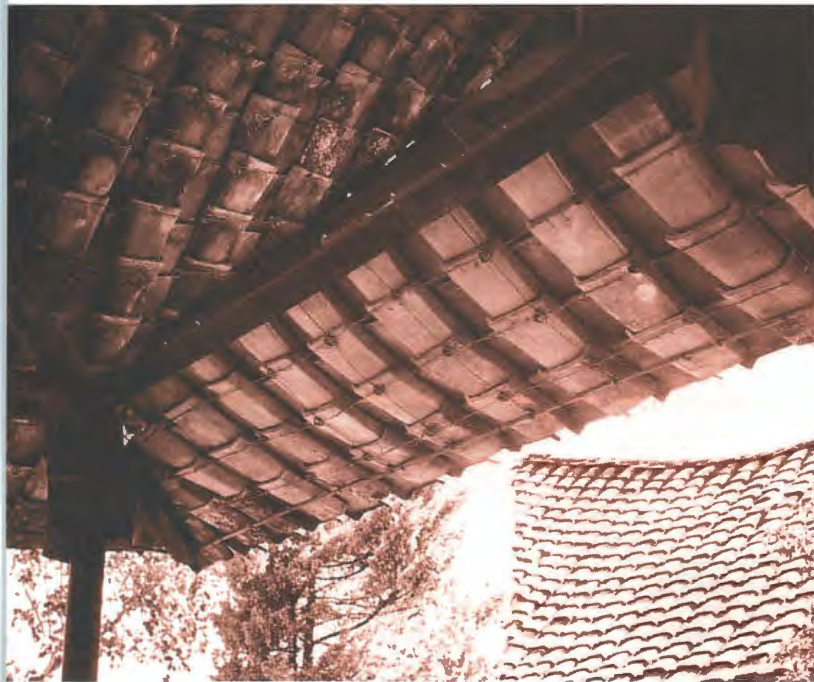
Fig. 2. View of a construction detail of Church at Pohsarang. Note how the roof tiles were held in place by the innovative tensile structure of the steel cable, instead of the usual timber rafters and battens
