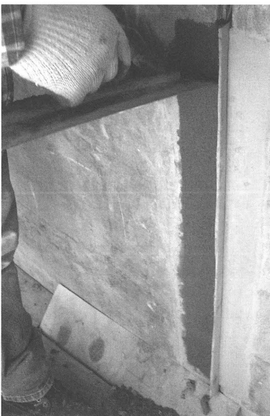
Fig. 7. Frank Lloyd Wright , Solomon R. Guggenheim Museum . In situ mock up for evaluation of repair products for concrete patch, New York, 2007
