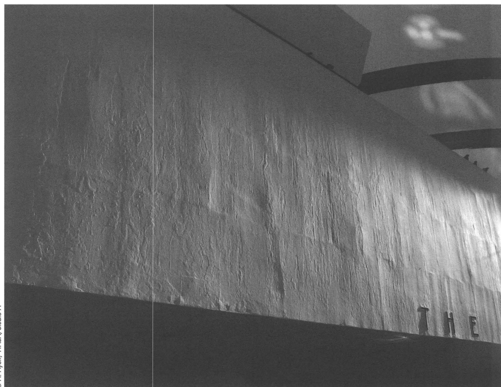
Fig. 2. Frank Lloyd Wright, Solomon R. Guggenheim Museum, façade. Surface texture and coating failures. New York City, 2004
