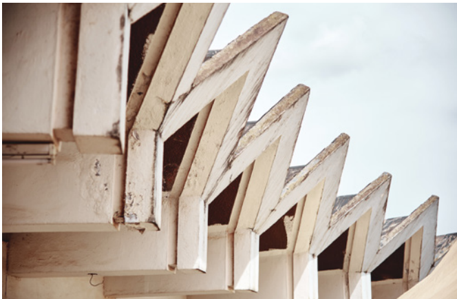
24 Roof details of the School of Fine Art and Industrial Design, Kyambogo University, Kampala, Uganda. © Timothy Latim, 2022.
