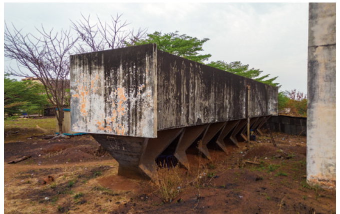
02 The water tower and tank, University of Nigeria Nsukka (Enugu Campus), Enugu, Nigeria. © Ikedi Chukwuka, 2023.
