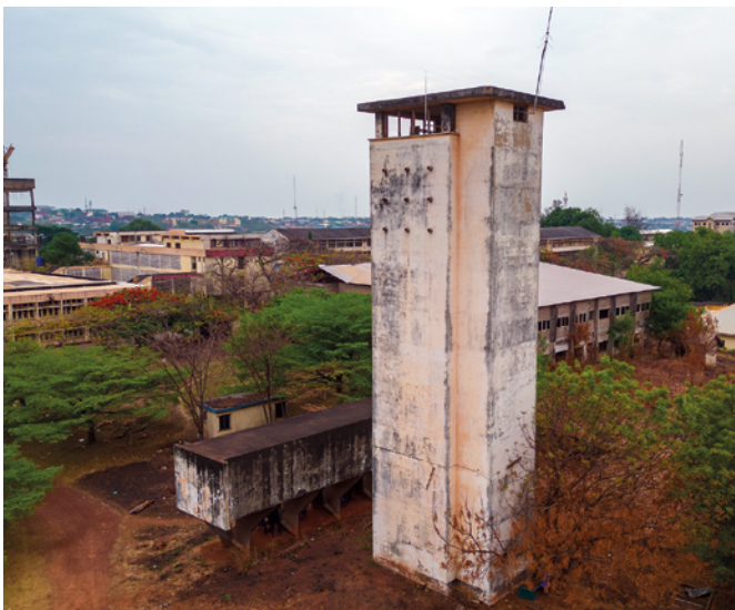
01 The water tower and tank, University of Nigeria Nsukka (Enugu Campus), Enugu, Nigeria. © Ikedi Chukwuka, 2023.
