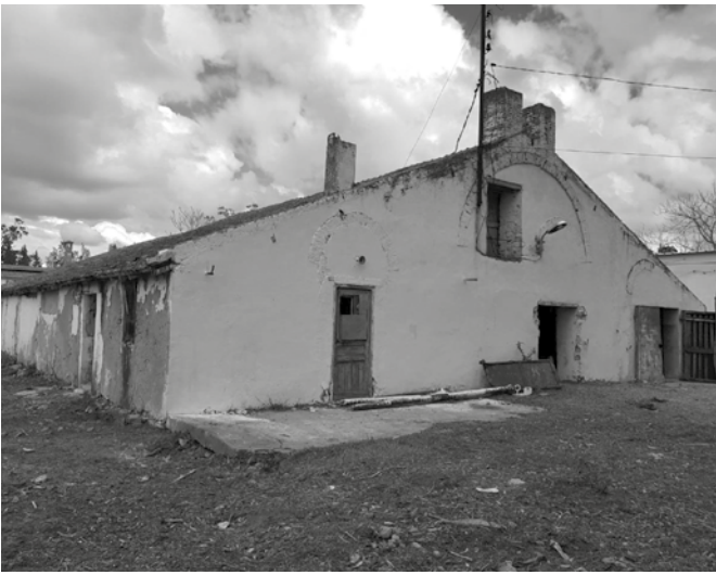
08 The dilapidated state of the annexes: the wine cellar and the chapel. © Author, 2023.
