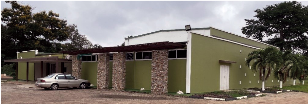
07 KCC after renovation, external view and inside view of closed court. © Author, 2023.
