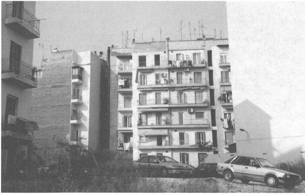
Characteristic interventions and problems: air-conditioning units, closed-in balconies, mechanised sunscreens, and damage through water infiltration and lack of painting.
