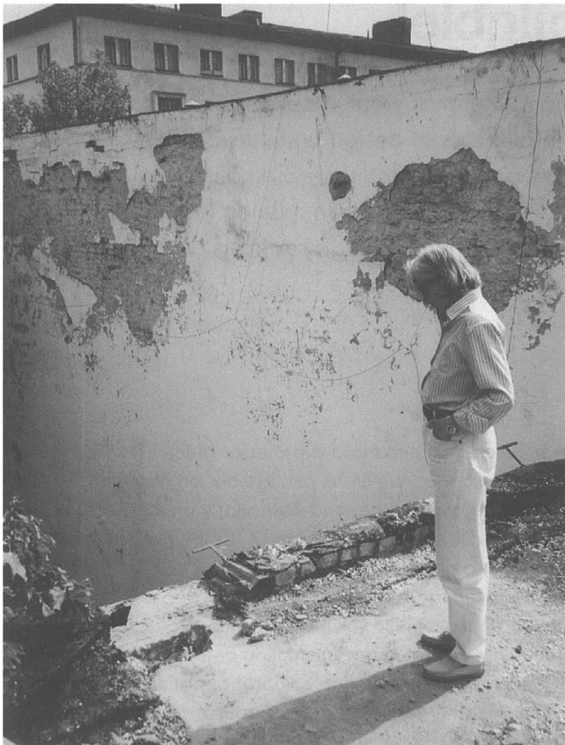
The lecture hall roof inspected by the Finnish team before repairs. All photos: Maija Kairamo.
