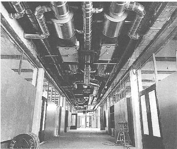
The amount of services packed between the lateral girders, before the vertical louvre ceiling was installed. Photo: Hans Vroege.
