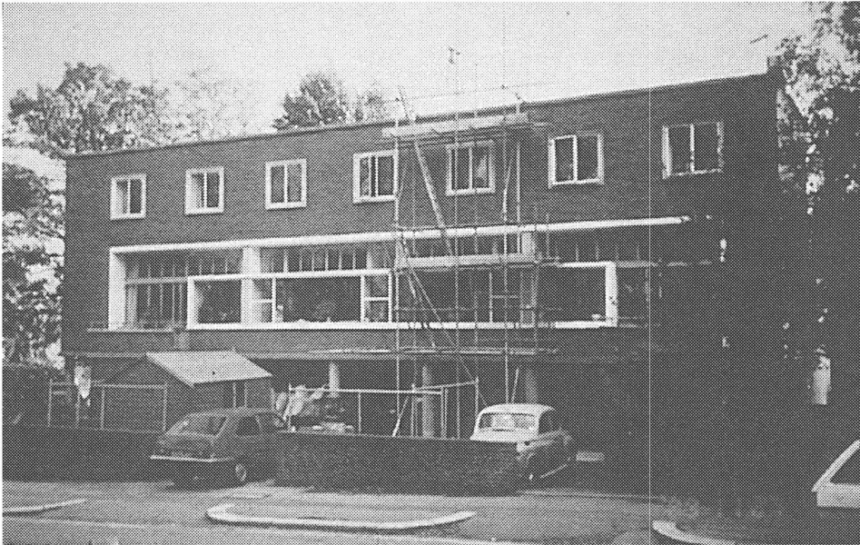
Willow Road, where the original ungalvanised steel windows have been sympathetically repaired in situ leaving the original glass in place.
