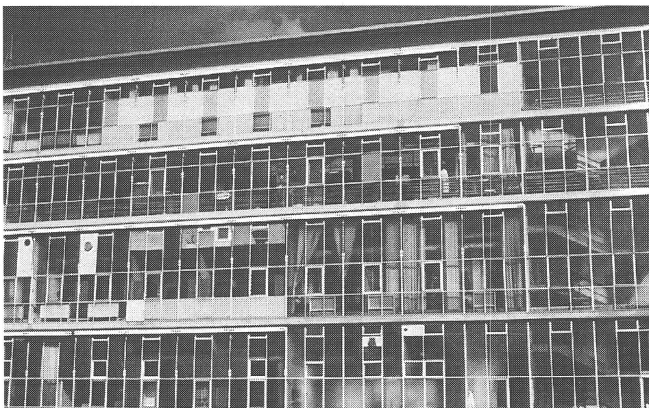
The 'D10' building before repairs were carried out, showing the original glazing and replacement hardboard, louvres, extract fans and blank panels.
