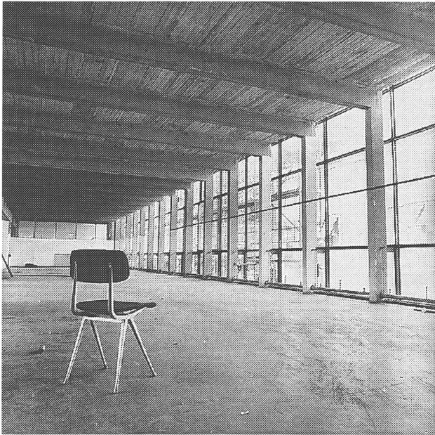
Empty school room with exposed concrete superstructure after removal of the false ceilings to increase thermal storing capacity. Photo: Hans Vroege.
