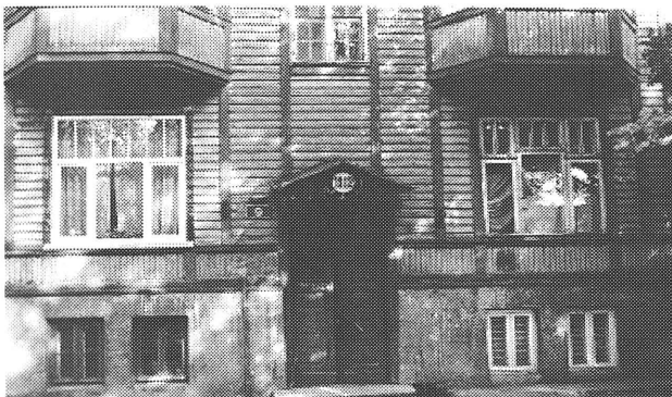
Pvc-u windows aesthetically compromise this 1912 traditional building in Tallinn's Koidula street.
