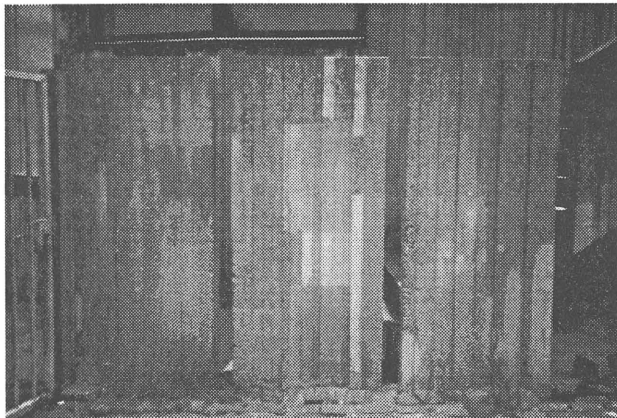
Test repairs by Sigma (left), Sika (middle) and Fosroc (right) showed a potential risk of patchwork effects, similar to previous at random repairs. Photo: Koos van der Zanden.
