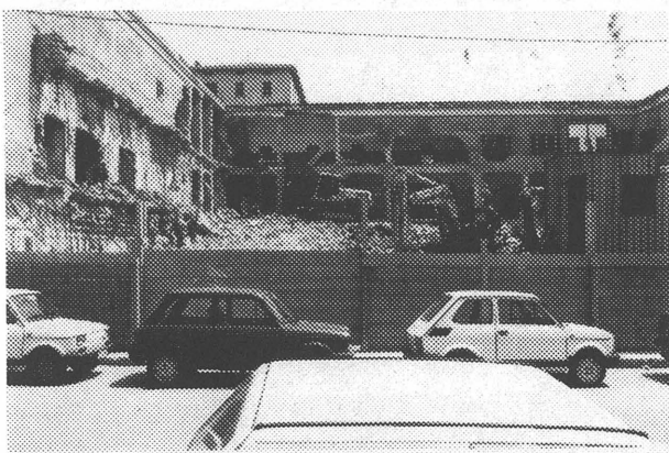
Bottom: the inner courtyard during demolition in 1992, to be compared with the far right photo on the previous page.
