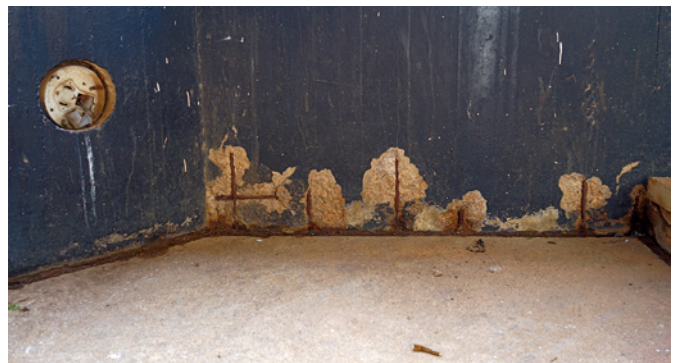
17 Obafemi Awolowo University, Assembly Hall, open corridor area, 2022. Damages to reinforced concrete surface due to insufficient concrete coverage. © Brenne Architekten, 2022.
