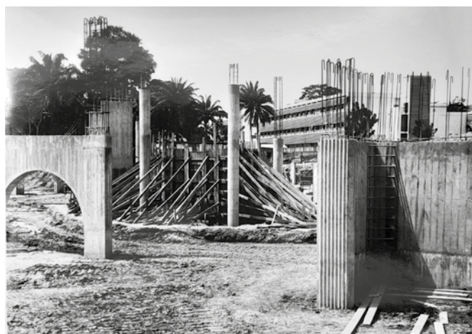
03 University of Ife, Assembly Hall, corrugated reinforced concrete column under construction, November 5, 1973. © Israel Kainy.
