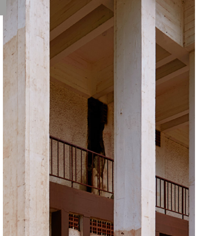
09 Leakage on level 01 on the Rukurato Hall, © Timothy Latim, 2023.
