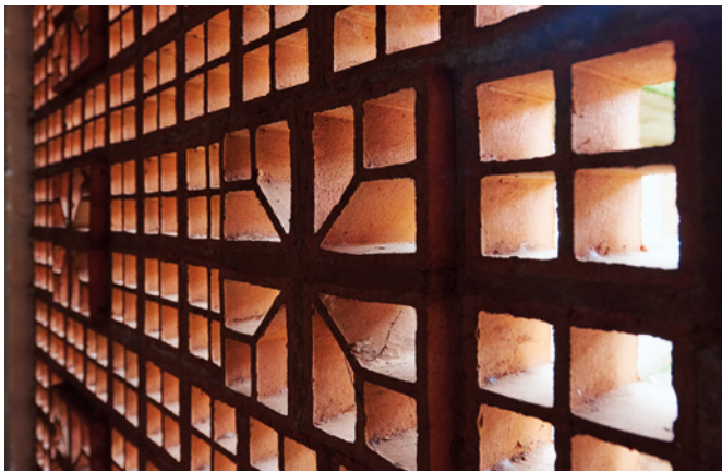
07 Detail of the hollow blocks at the east and west facades of Rukurato Hall. © Timothy Latim, 2023.
