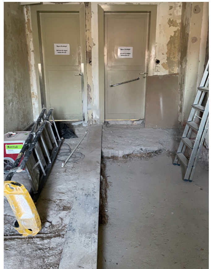
07 The local intervention and exposed layers of Solomite and aerated concrete materials in the library's uppermost floor in the 1932 western wing. © Marcelo Rovira Torres, 2022.
