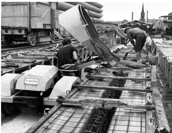
02 Keith Ingham for BDP, Central Bus Station and Car Park, Preston, Lancashire, England, 1969, construction site. © Historic England Archive. John Laing Photographic Collection, c1969
