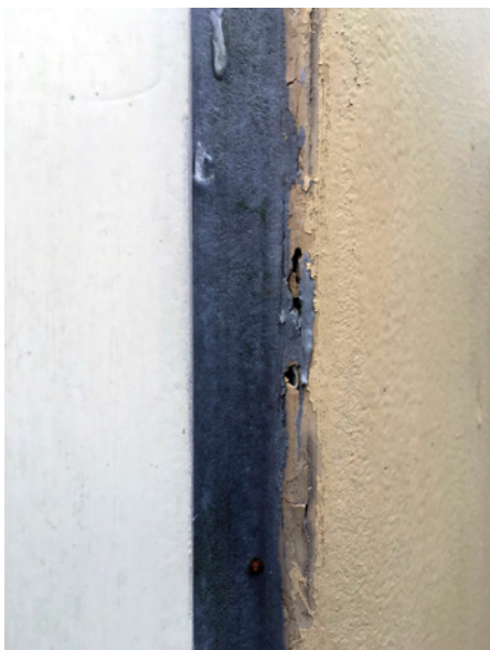
04 Corner voids due to an absence of glass fibre matting behind the outer gel-coat layer at the Olivetti Building, December 2018. © R. Loader
