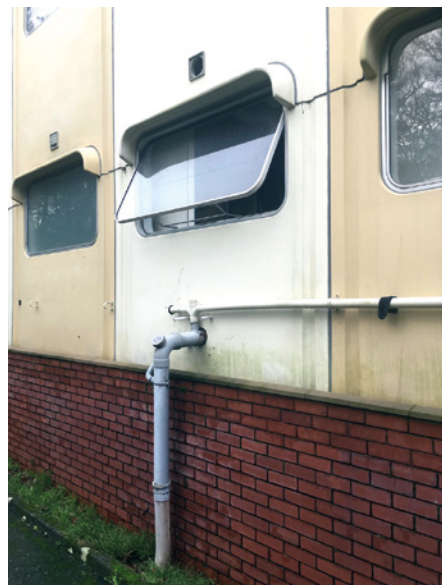
03 Drain-pipes and vents cut through a GRP panel at the Olivetti Building, December 2018. © R. Loader
