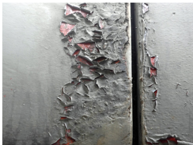
07 Detail of the deterioration of the exterior top coat in 2019 that had been applied during the restoration of the Futuro house in 2009. © E. Stamatopoulou, 2019
