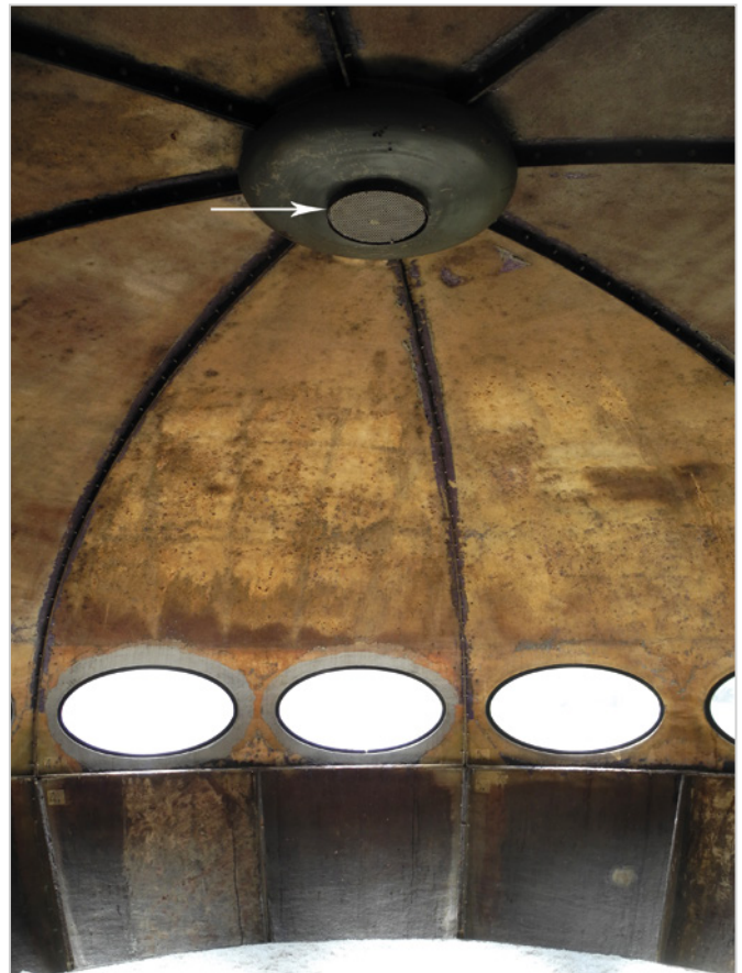
11 Interior of the Futuro house. The arrow indicates the position of the air-conditioning. © E. Stamatopoulou, 2015
