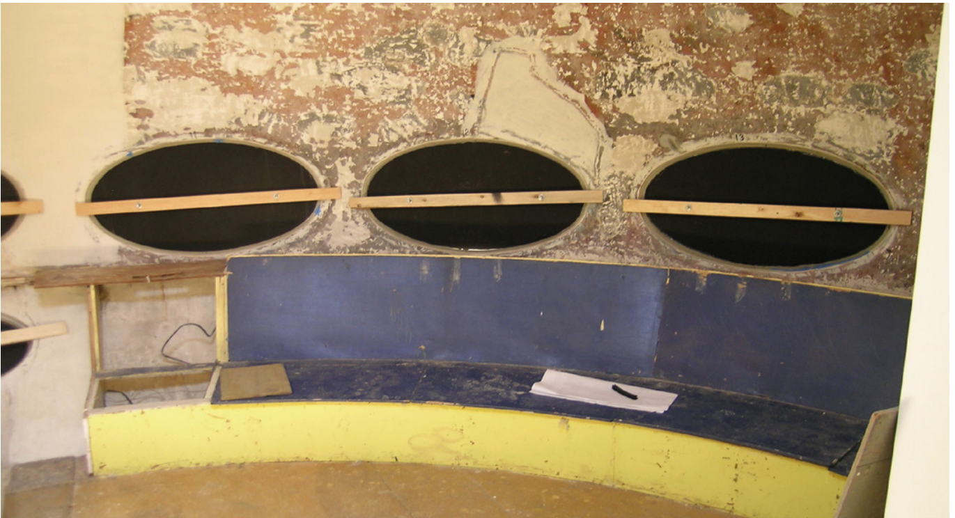
08 Interior of the Futuro showing the interior damages, missing windows and bench seat sitting area. © M.W. Donaldson, August 15, 2006
