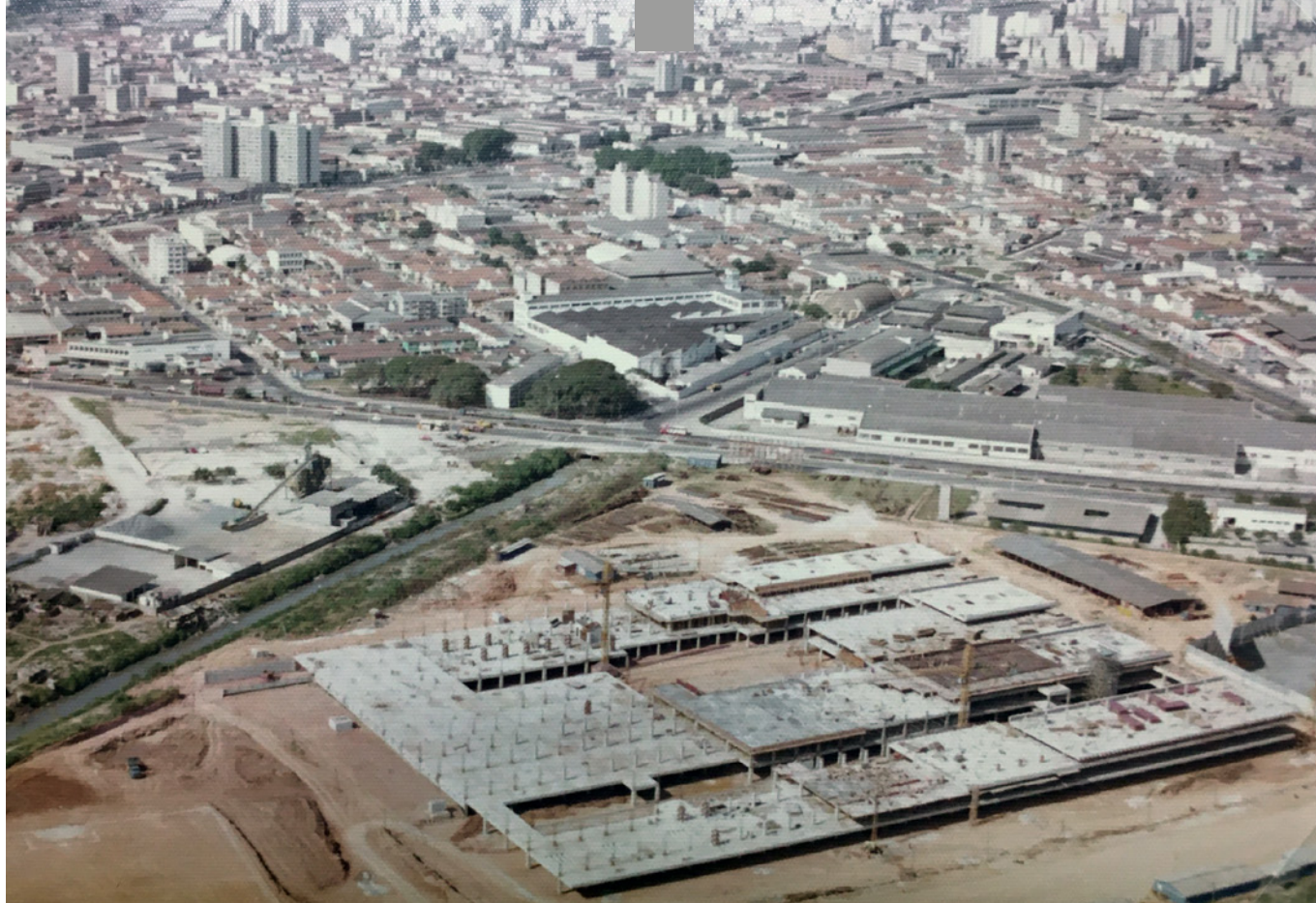
01 Santa Casa Teaching Hospital: The gigantic structure under construction, early 1970s. © Fábio Penteadó's Archive, 2022.
