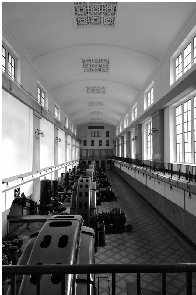
04 E. Faesch, Power House, Fala hydropower plant, 1918, with an innovative inside shell ceiling, only 5 cm thick, has been renovated into a museum, partly still operating with new generators. This is a case of symbiosis between heritage protection and the industry. © Miran Kambič.
