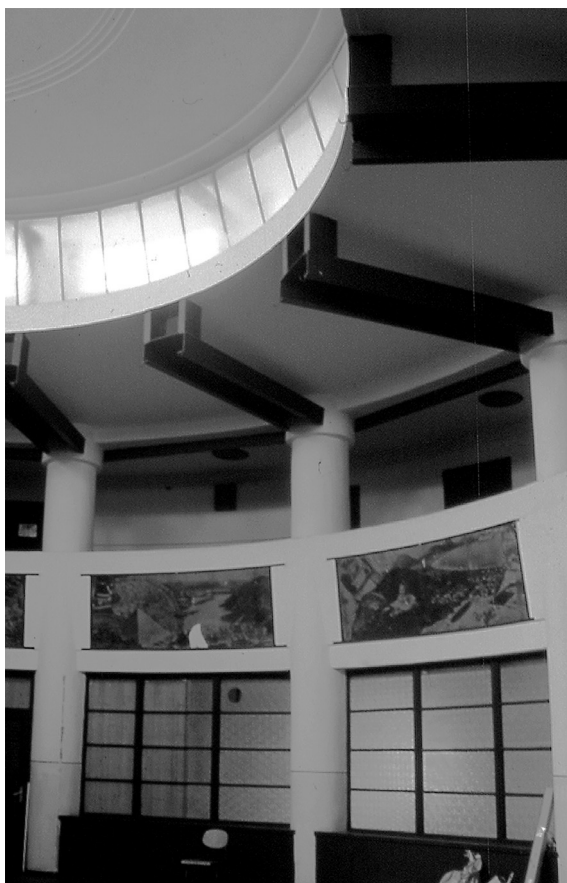
04 Virgil Bierbauer and László Králik, Public airport, Budaörs, Hungary, 1935-1937. Reinforced structure of the passenger hall. © Ferkai András, 2001.
