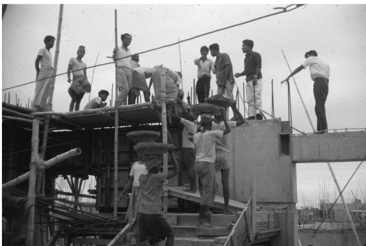
02 Louis Kahn, National Assembly Building of Bangladesh, Dhaka, 1964-1982. © Harry Palmbaum Collection, The Architectural Archives, University of Pennsylvania.
