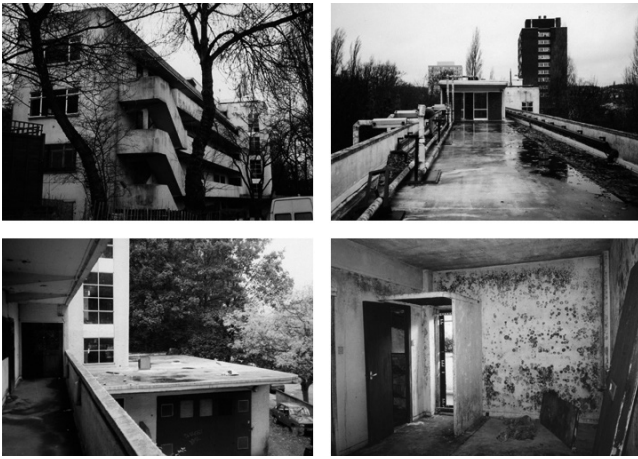
06 Wells Coates, Lawn Road Flats (The Isokon), London, UK, 1933-34. Condition before restoration work began. © Avanti Architects, 2000.
