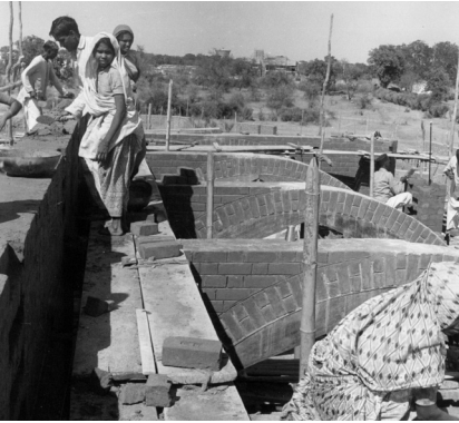
01 Louis Kahn, Indian Institute of Management in Ahmedabad, India, 1962-1974. Construction of dormitories. © UPENN Archives, SNK, 1960s.
