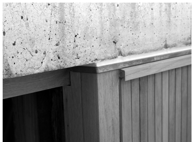
09 Louis Kahn, Salk Institute, La Jolla, California, USA, 1959-1965. Folded metal flashing installation at top of window. © Wiss, Janney, Elstner Associates, Inc. 2016.
