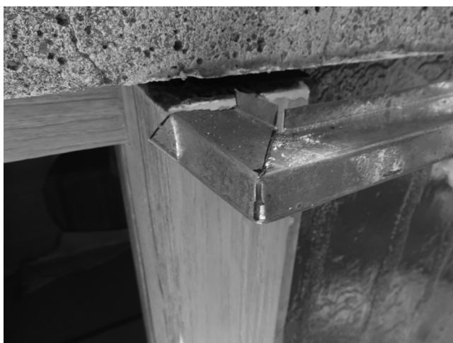
08 Louis Kahn, Salk Institute, La Jolla, California, USA, 1959-1965. New metal flashing at top of window. © Wiss, Janney, Elstner Associates, Inc. 2016.
