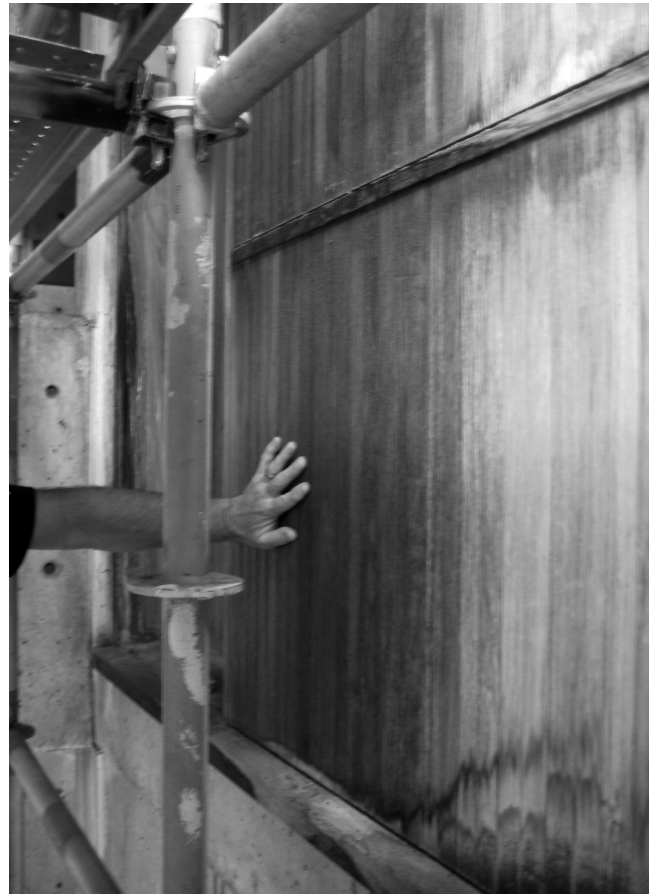
07 Louis Kahn, Salk Institute, La Jolla, California, USA, 1959-1965. Treatment discoloration and varied weathering patterns. © Wiss, Janney, Elstner Associates, Inc. 2015.
