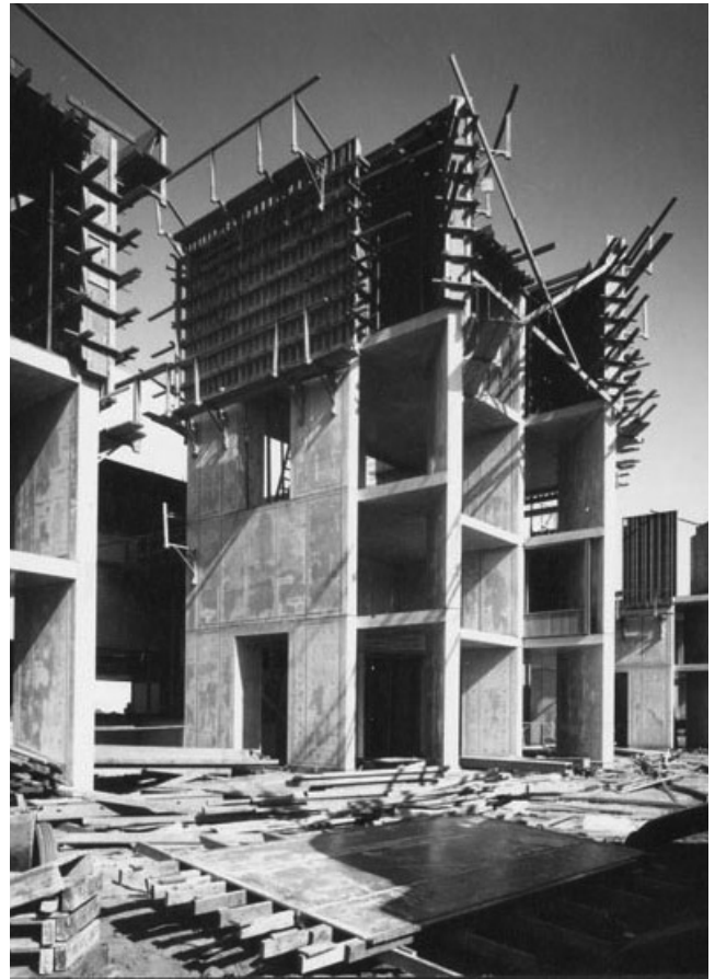
05 Louis Kahn, Salk Institute, La Jolla, California, USA, 1959-1965. Under construction. © Louis I. Kahn Collection, University of Pennsylvania and the Pennsylvania Historical and Museum Commission.
