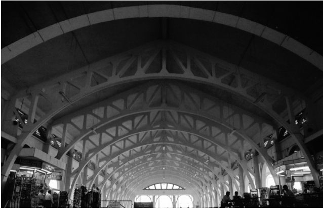
03 Public Works Department, Clifford Pier, Singapore, 1933. Interior view showing the reinforced concrete arched trusses. © Jonathon Lin, goo.gl/Zb2Pov, used under CC license.
