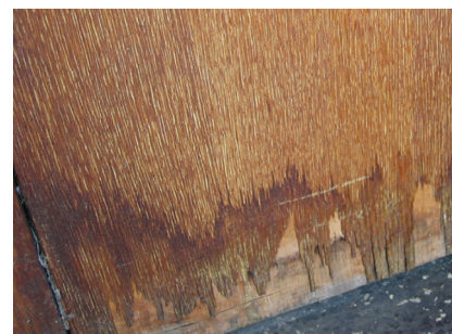
05 Mies van der Rohe, Carr Memorial Chapel, Chicago, Illinois, 1952. Damage at the bottom of wood veneer panel due to improper cleaning methods and UV degradation. © Harboe Architects, 2011.
