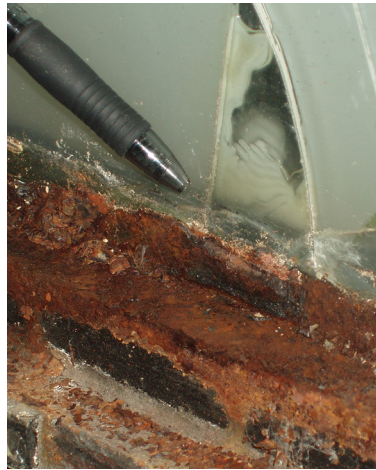
07 Mies van der Rohe, Crown Hall, Chicago, USA, 1950-1956. Detail view of sill with glazing stop removed. © Krueck + Sexton, 2005.
