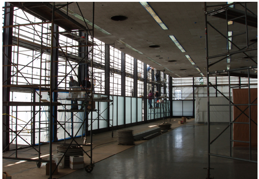
05 Mies van der Rohe, Crown Hall, Chicago, USA, 1950-1956. Restoration works. © Krueck + Sexton Architects, 2005.
