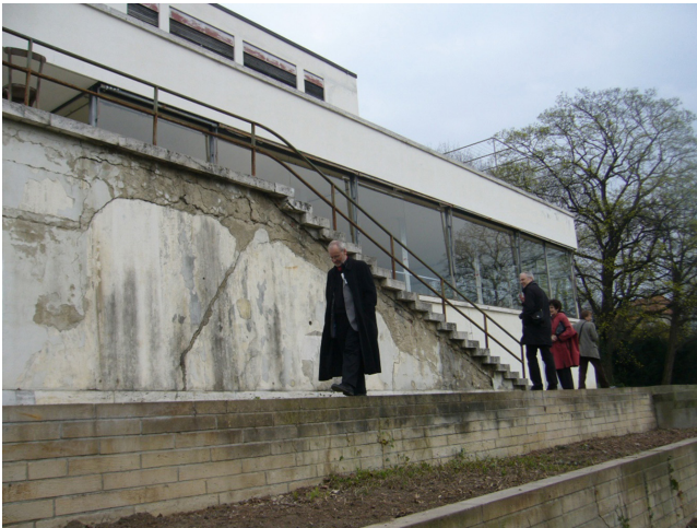
08 Mies van der Rohe and Lilly Reich, Tugendhat House, Brno, Czech Republic, 1929-30. Garden stair case, before restoration: stability problems and rests of original façade plaster and later coatings, garden walls reconstructed in 1970 using carved stones. © Ana Tostões, 2009.
