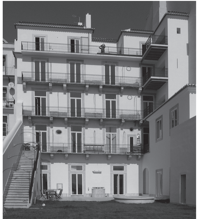
09 Souza Oliveira Arquitectura & Urbanismo, in collaboration with João Botelho, Rua de São Mamede 15, 3 rd floor, Lisbon, Portugal, 2006. Back Façade with balconies. © Alberto de Souza Oliveira.
