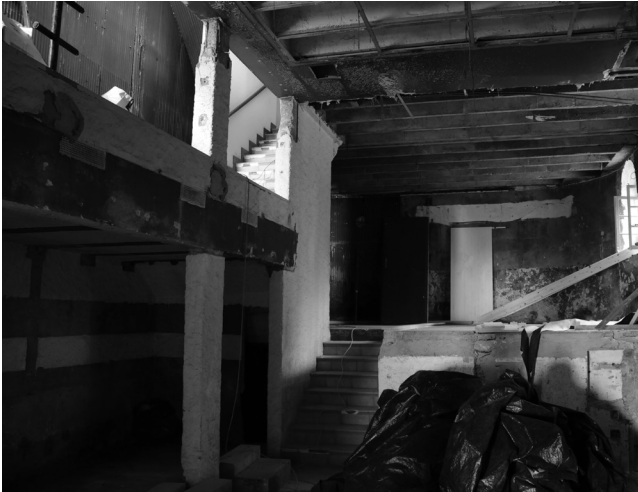
08 Alberto Sartoris, Cercle de l'Ermitage , Epesses, Switzerland, 1935. Bar. The undergoing demolition work has revealed an unexpected amount of original elements © JC Dunant, 2012.
