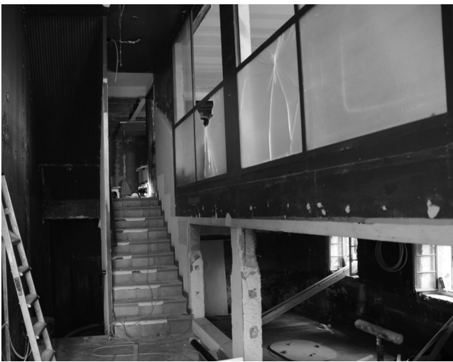
10 Alberto Sartoris, Cercle de l'Ermitage , Epesses, Switzerland, 1935. Gallery. The undergoing demolition work has revealed an unexpected amount of original elements © JC Dunant, 2012.
