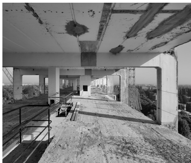
04 Willy Van Der Meeren, Ieder Zijn Huis , Brussels, Belgium, 1953-1961. A typical storey dismantled during renovation. © ORIGIN, Georges De Kinder.
