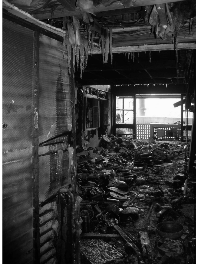
03 Le Corbusier, Unité d'Habitation , Marseille, France, 1945-1952. One of the apartments most damaged by the fire. © Photo F. Bolton/ssea, February 2012. FLC/2016, Prolitteris, Zurich.
