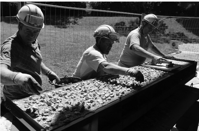
04 Le Corbusier, Unité d'Habitation , Marseille, France, 1945-1952. Work on restoration of the east façade. Prefabrication on site of the reinforced concrete cladding of the loggias. © Photo F. Bolton/ssea, November 2015. FLC/2016, Prolitteris, Zurich.
