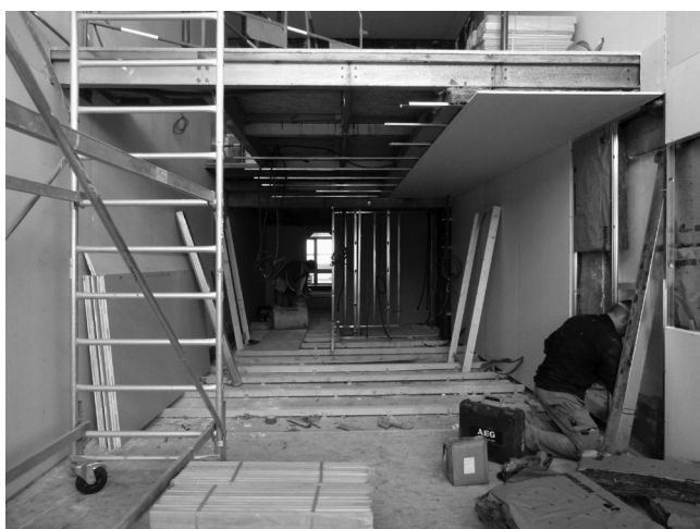
06 Le Corbusier, Unité d'Habitation , Marseille, France, 1945-1952. Reconstruction of fire-damaged apartments. Installation of the firewall partitions of precast gypsum panels. © Photo F. Botton/ssea, March 2014. FLC/2016, Prolitteris, Zurich.
