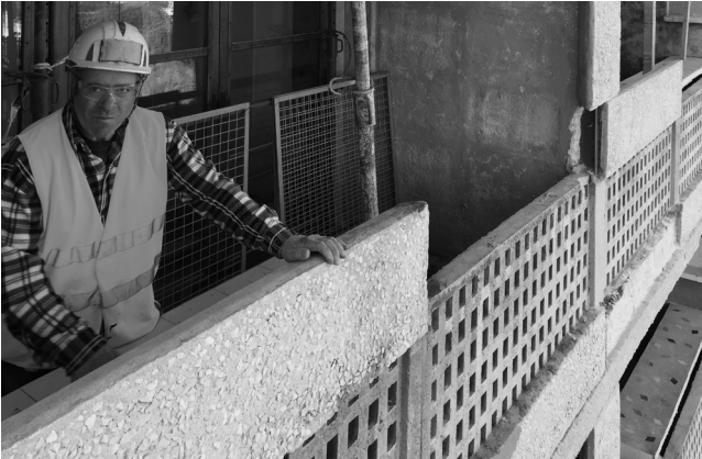
02 Le Corbusier, Unité d'Habitation , Marseille, France, 1945-1952. Work on restoration of the east façade. Replacing the prefabricated cladding of the loggias rebuilt identically. © Photo F. Bolton/ssea, November 2015. FLC/2016, Prolitteris, Zurich.
