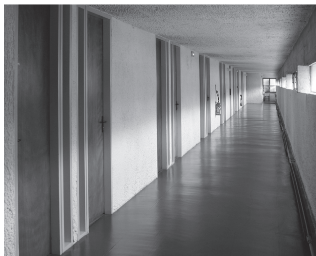
08 Le Corbusier, Couvent de La Tourette , Eveux, France, 1953-1960. The fire detection system doesn't change the original appearance of the cell corridors. © FLC/SPA, Roberta Grignolo.
