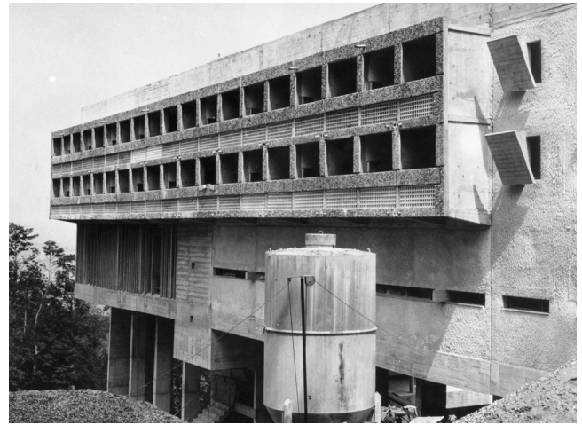
02 Le Corbusier, Couvent de La Tourette , Eveux, France, 1953–1960. The cracks on the acrotères (parapets) are already visible before the completion of the worksite. © FLC/SPA, ACT, late 1950s.
