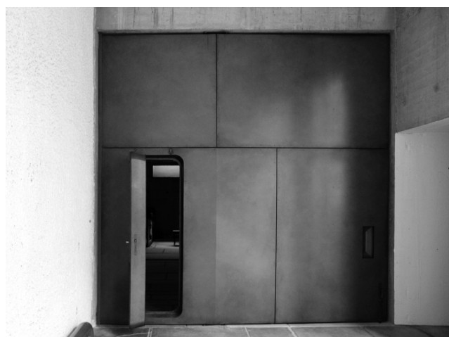
05 Le Corbusier, Couvent de La Tourette , Eveux, France, 1953-1960. South church pivot door built by Mortamet in 1989 following the unbuilt 1959 design of Le Corbusier. © FLC/SPA, ACT, Roberta Grignolo.
