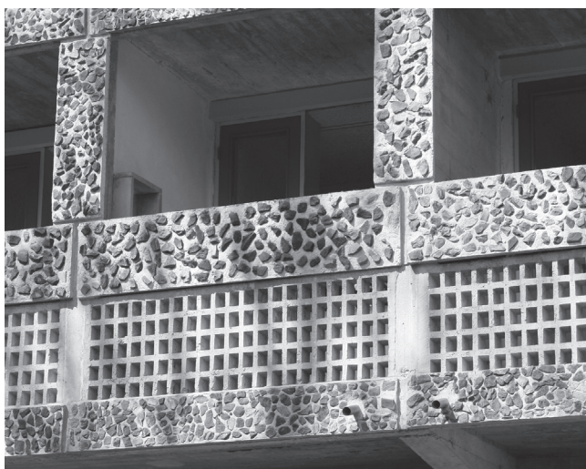
07 Le Corbusier, Couvent de La Tourette , Eveux, France, 1953-1960. View of the loggias with the wiring ducts running in the goulotte above the window fixtures. © FLC/SPA, Roberta Grignolo.
