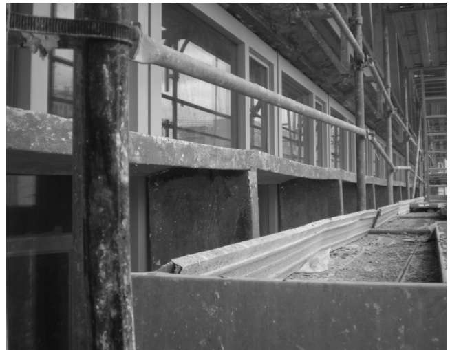
10 Le Corbusier and Pierre Jeanneret, Cité de Refuge , Paris, France, 1933. Installation of timber window frames painted in yellow. © Gilles Ragot, January 2015.
