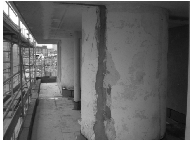
08 Le Corbusier and Pierre Jeanneret, Cité de Refuge , Paris, France, 1933. The construction work on the 7 th and 8 th floors permitted a return to the original interior and exterior volume of the director's apartment. © Gilles Ragot, January 2015.
