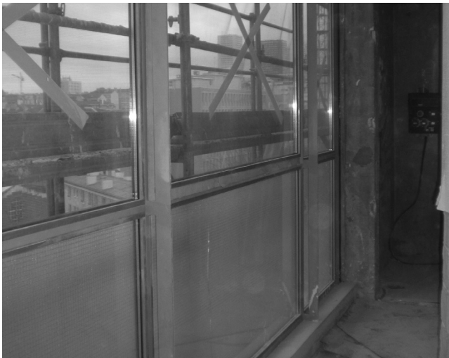
09 Le Corbusier and Pierre Jeanneret, Cité de Refuge , Paris, France, 1933. To restore the profiles of metal frames of the 7 th floor, as closely as possible to the original, a solution of invisible interior vertical stiffeners was adopted. © Gilles Ragot, January 2015.
