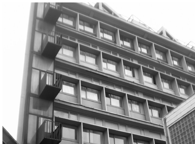
04 Le Corbusier and Pierre Jeanneret, Cité de Refuge , Paris, France, 1933. South façade before the last restoration work. On the left-hand side the slice of the original 1933 glass facade and the balconies redone at an unknown date, though after the death of Le Corbusier. © Gilles Ragot, 2012.
