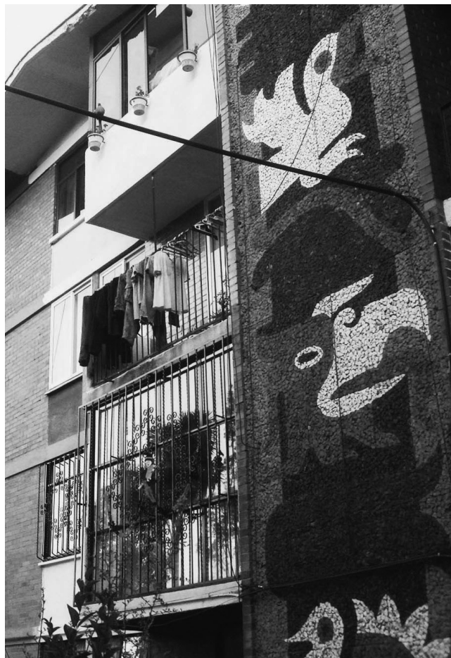
02 Alejandro Prieto, José María Gutiérrez & Pedro Miret, Independence Social Services and Housing Unit, Mexico City, 1960. 4-floor apartment block façade. © Juan Pablo Rodríguez Méndez, 2010.
