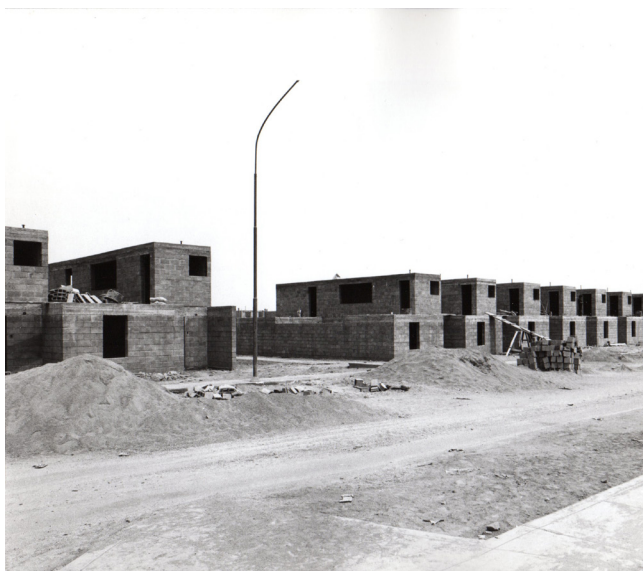
10 Kikutake, Kurokawa & Maki, PREVI , Lima, Peru, 1960s. Houses under construction. © Peter Land, 1970.
