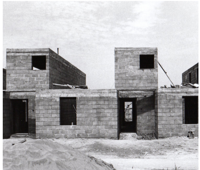
09 Kikutake, Kurokawa & Maki, PREVI , Lima, Peru, 1960s. Houses under construction. © Peter Land, 1970.
