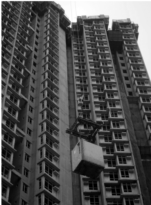
11 Construction of site-specific 45-storey blocks of HKHA public rental housing underway at Kai Tak Site 1a, Kowloon, in 2012: this view shows a prefabricated services unit (bathroom/kitchen) being winched up. © Miles Glendinning, 2012.
