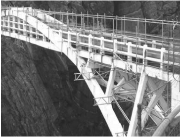
Figure 1. Temporary access scaffold supported directly from the arch ribs erected in June 2005.
